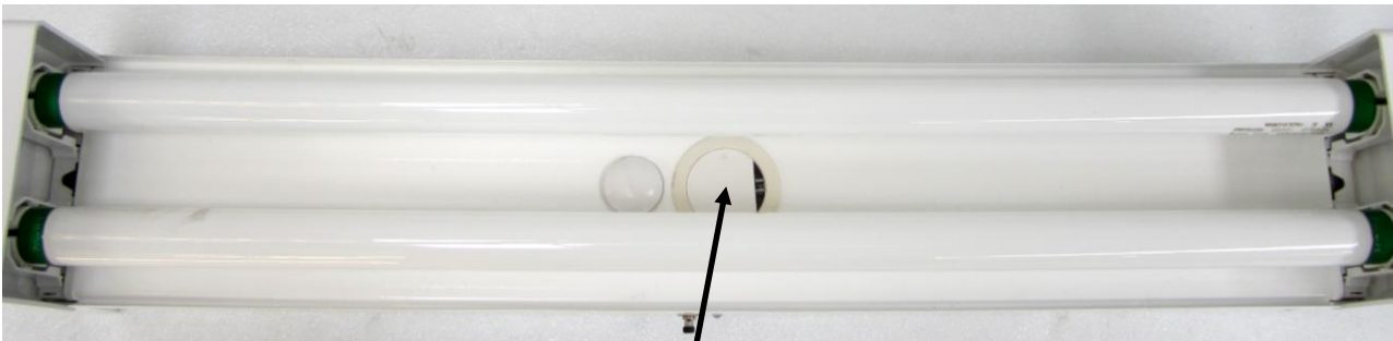
Typical Sensor Location: 2 x 18W Batten
